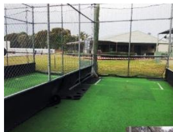
Photo left: Cricket nets showing single faced chain wire / damaged rubber side mats.
