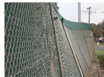
Photo: Tennis court fence which seemingly wasn't engineered to allow for local wind gusts.
